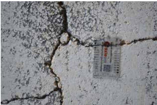
Crack Measured with Mil Gauge
