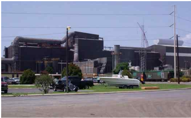
View of the completed project. Approximately 140,000 sq ft of surface was cleaned and painted to match the new addition (at right, with white stripe).
